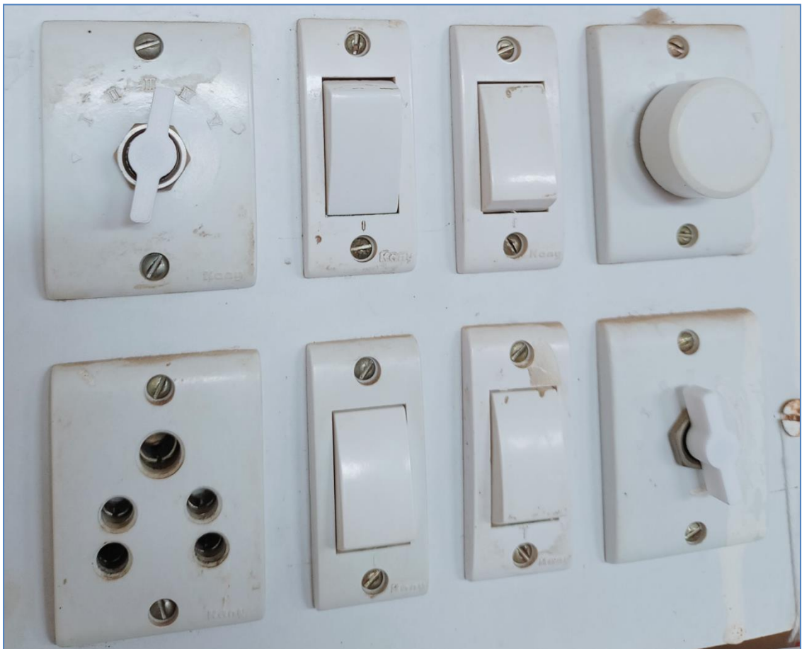
Broken Fan Regulators are replaced with 3D printed Regulators
